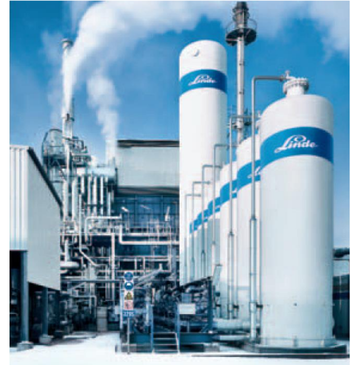
Steam reforming plant in Brunsbüttel (Linde AG)
